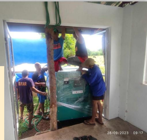
Installation of Filtration System and Generator Set at the Legislated Hatchery in Bantayan Island, Cebu
